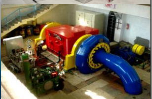
Hydro Turbine Generator & Site Installation
