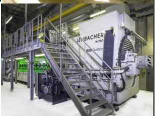
Gas Engine Generator & Site Installation
