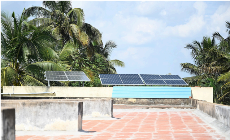
Solar panels on rooftop
