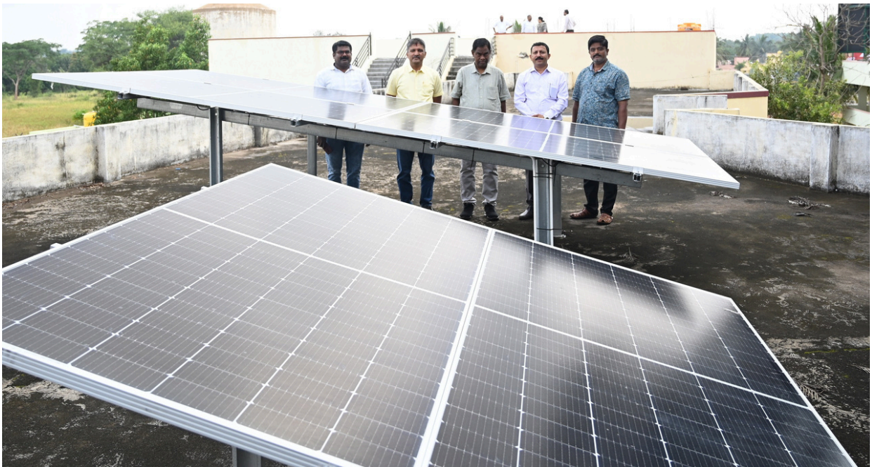
Solar panels on rooftop at Yantaganahalli
